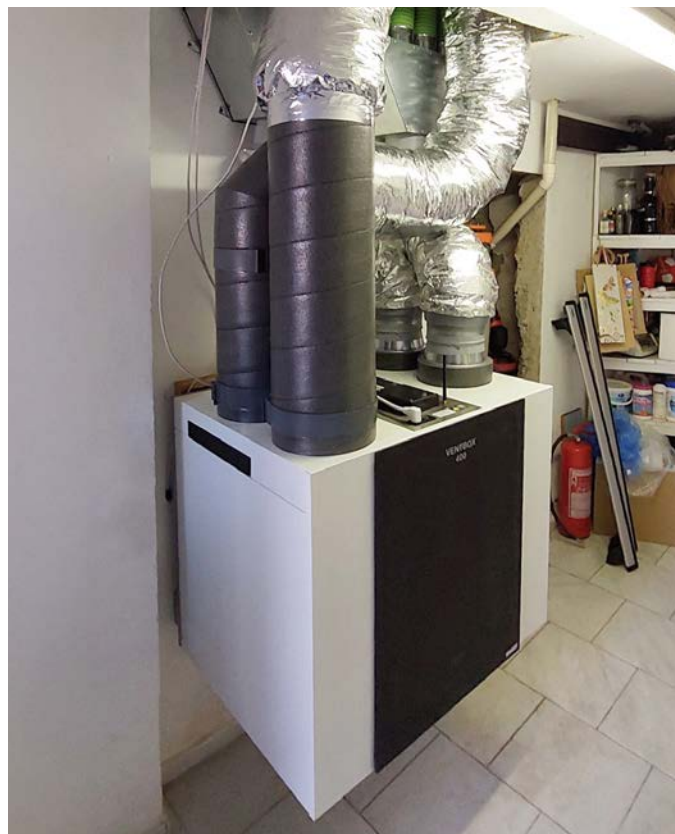
Installed VENTBOX 400 unit in the utility room
